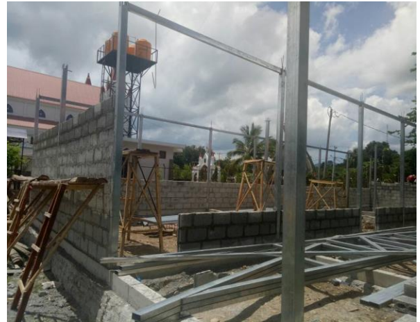
Construction began in January this year and the building is expected to be completed in time for second term. St Esteveo Catholic school is located alongside the Vqq church.
