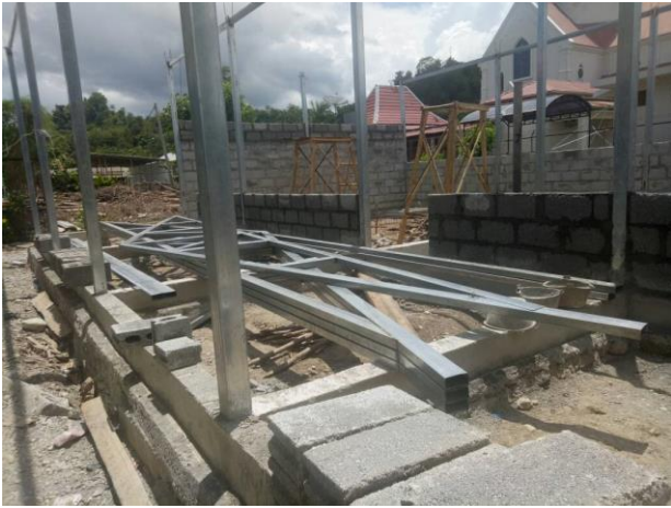
St Mary's Geelong has provided the finance for building 3 new classrooms at St Esteveo Catholic school. The school has recently enrolled 60 new students!
