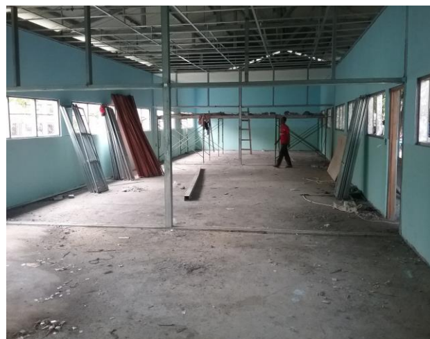
St Mary of The Angels, Geelong, is building 3 new classrooms at St Estevao Senior Secondary school. The building project is nearing completion.
